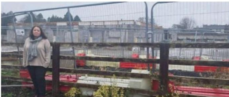
Sensational Kids founder Karen Leigh at the construction site for the National Child Development Centre which has now ground to a halt
